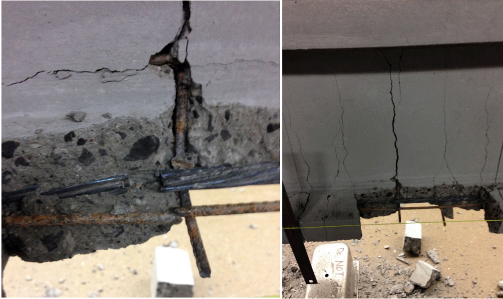
Figure 14: Ultimate Failure (Strand/Crack)
