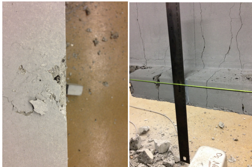
Figure 15: Crushing / Visual Indication of Deflection
